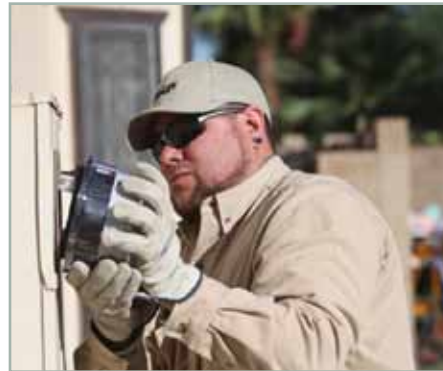
Meters automatically register on the system within minutes of installation
